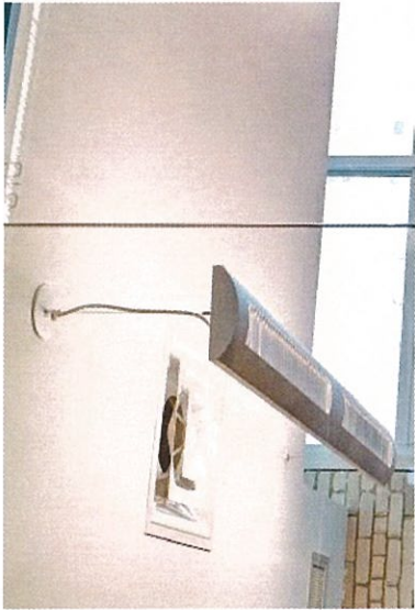
LED FIXTURE ABOVE WORKSTATIONS
